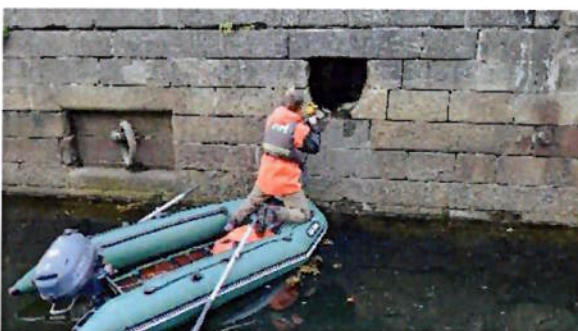
Plate 8.23 Inspecting known otter holt for spraint at the MV Cill Airne on the River Liffey estuary
