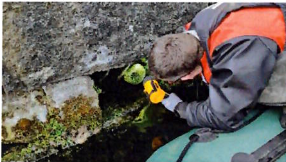
Plate 8.13 Inspecting an spraint site in quay wall via boat at Grand Canal Dock
