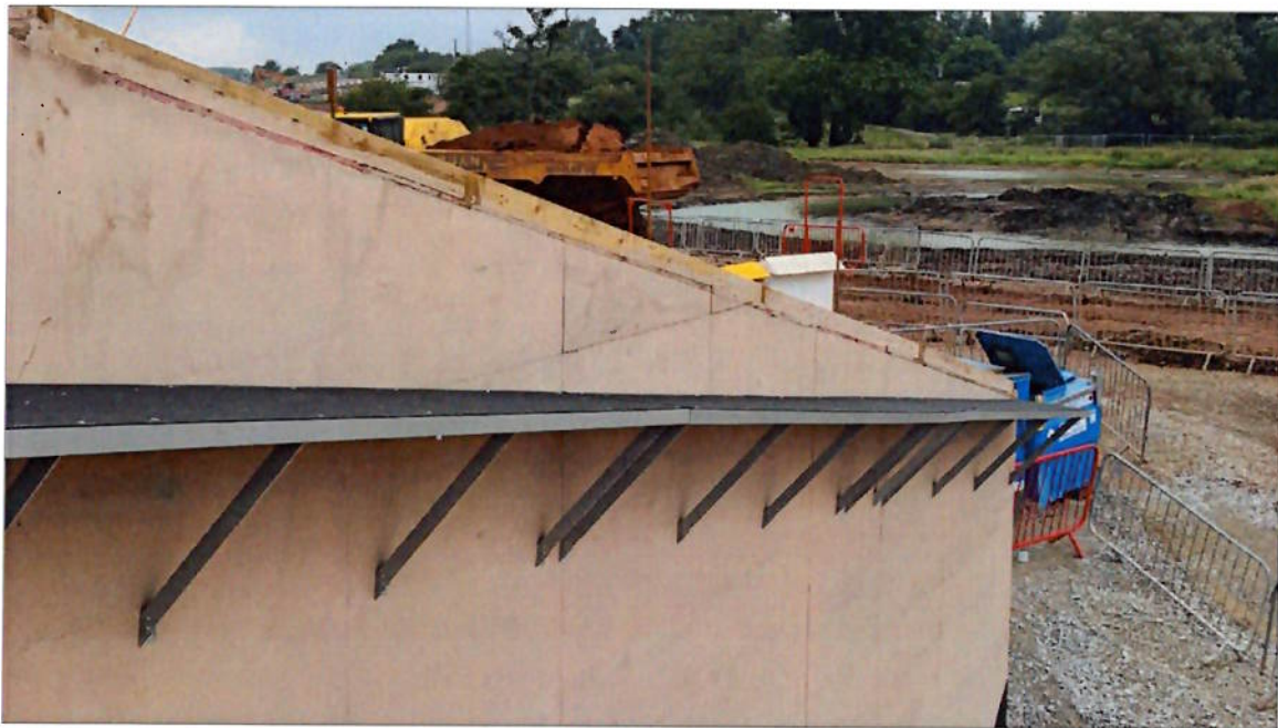
Plate 5.5 Another example of bolt-on mammal shelf/ledge for otter passage at a large road culvert (source: Althon, UK)
